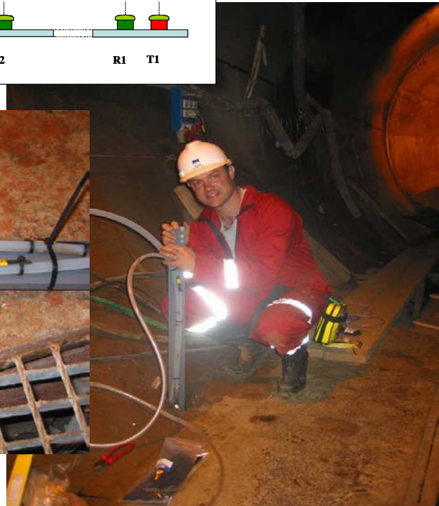
Figure 6-1: Top: Schematic diagram of the locations of all transducers on a single frame. Left: Photo of a section of the transducer assembly. Right: The transducer assembly during installation.
